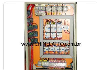
Electrical control panel of BH-200 boring machine with contactors, relays and wiring system
