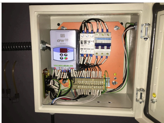
Detail — Electrical panel with CFW10 inverter and contactors for RVC-1000M grinder control
