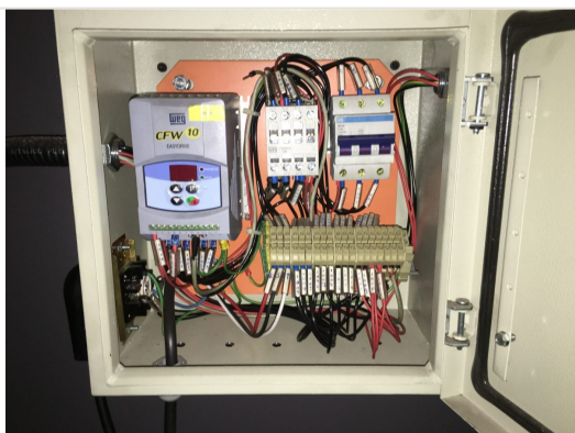
Detail — Electrical panel with CFW10 controller, contactors and control system for crankshaft grinder
