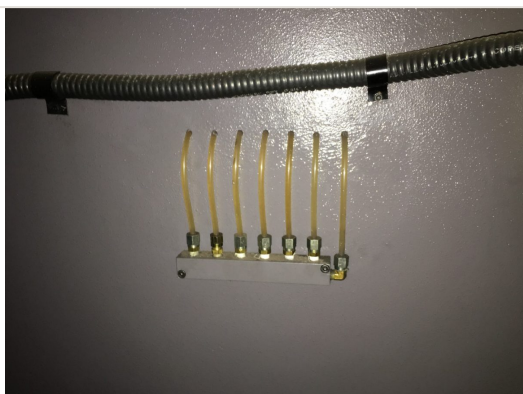
Detail — Bed lubrication distribution system with 7 yellow tubes connected to distributor block
